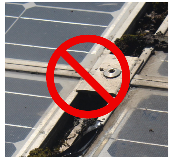
Typical example of delamination caused by algae growth between the frame and the laminate 5
