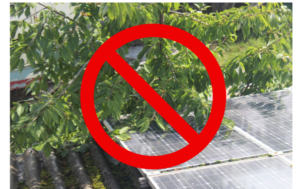
Growing plants lead to shadows on the cells: Hot spot risk, loss of performance 5
