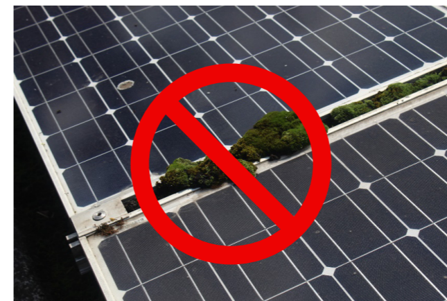
Algae growing in wet conditions destroy the insulation 4
